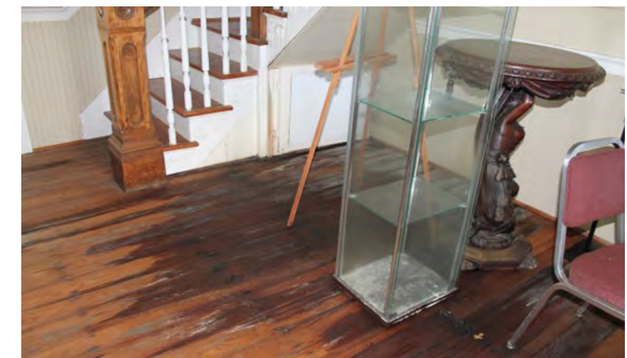
Interior view of water damage on floor near staircase
