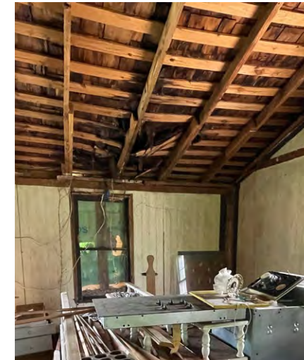
Damaged roof detail
