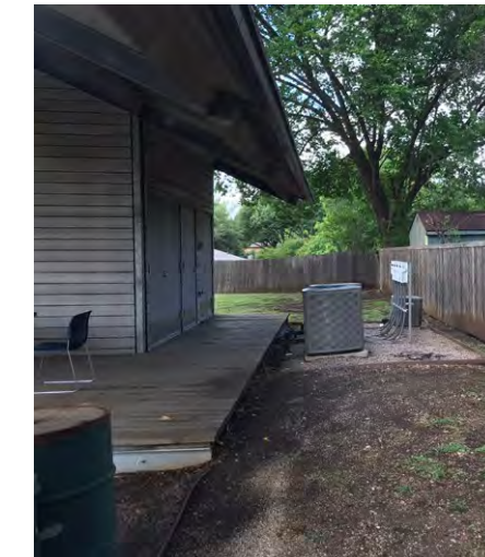
AC units located north of structure, view facing west
