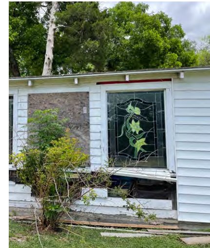
Damaged wall of connecting hallway
