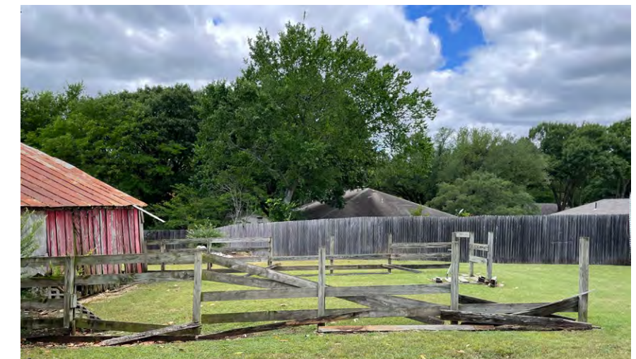
Deteriorating fence north of barn
