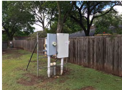
Electrical service, view facing northwest
