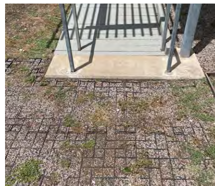
Left: Ramp leading to new restroom detail, view showing grid-paver on parking lot driveway
